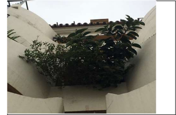
DRAINS RISK TO TERRACE BELOW
