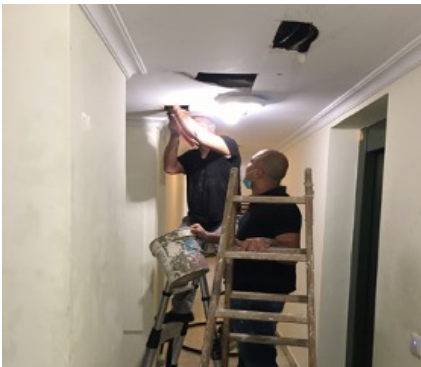
This photo illustrates a very amateurish approach to a serious incident. Over a period of 5 weeks this pipe burst 4 times, causing extensive flooding into the lift shaft, stairways, & 3 storage rooms below. Today we still await an 'emergencies protocol' from Meridional on what an owner must do in such circumstances
